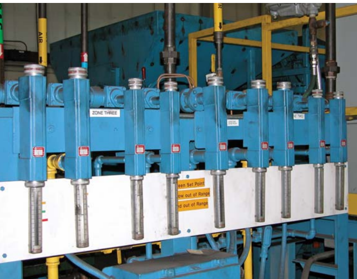
Fig. 1. Typical flow control panel (multiple-zone continuous furnace)
