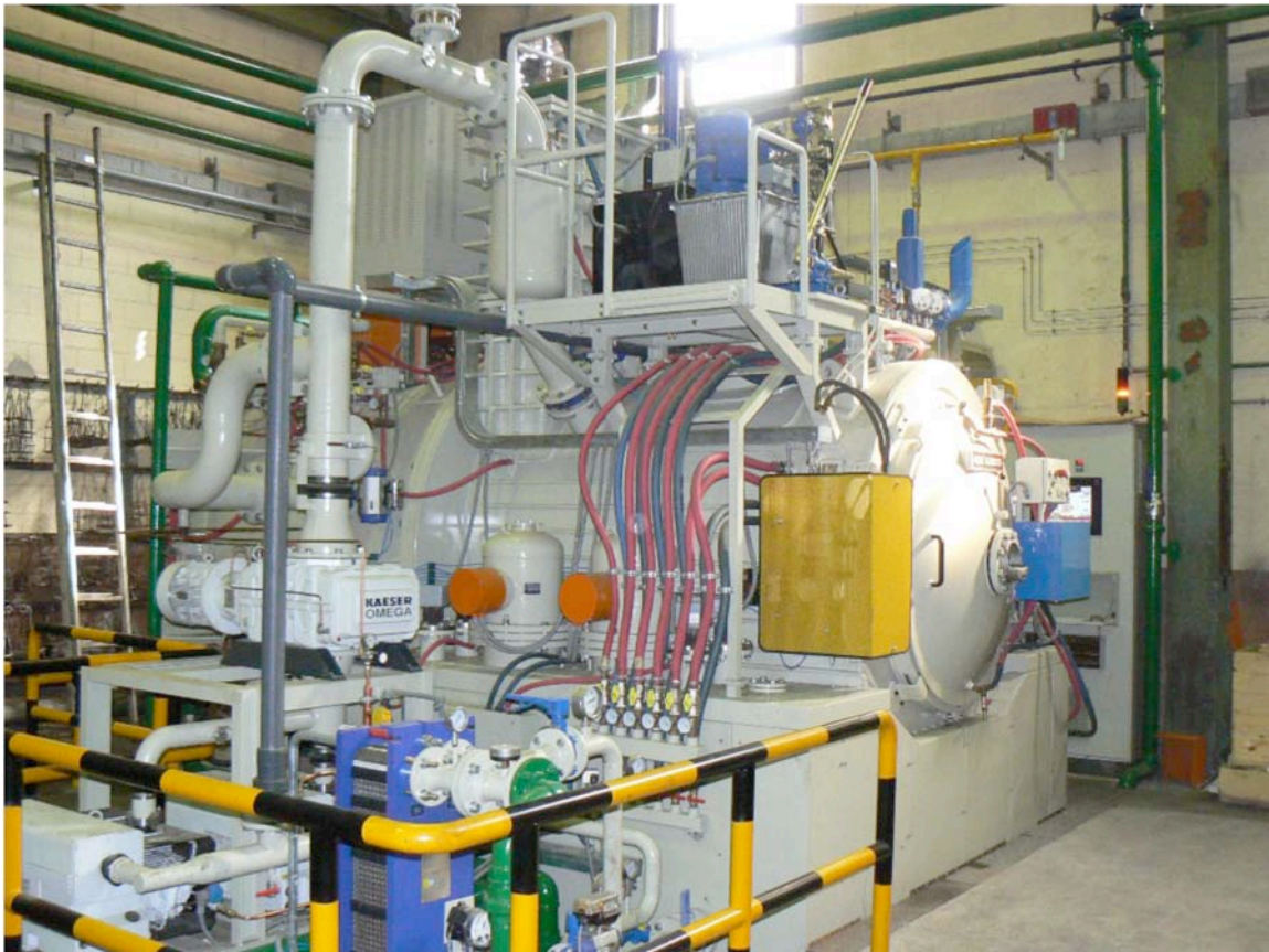
Figure 5 Typical Dual Chamber Horizontal Vacuum Oil Quench Furnace (Photograph Courtesy of SECO/WARWICK Corporation)
