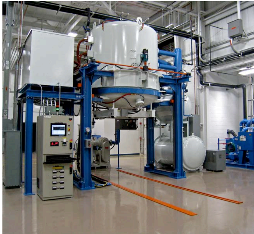
Figure 16 Modern Vacuum Furnace Controls
